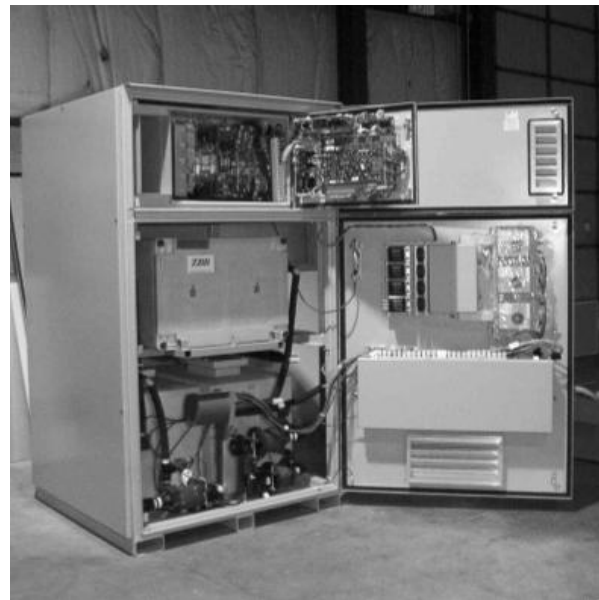
Fig. 5: Battery/PCS enclosure with door open.
