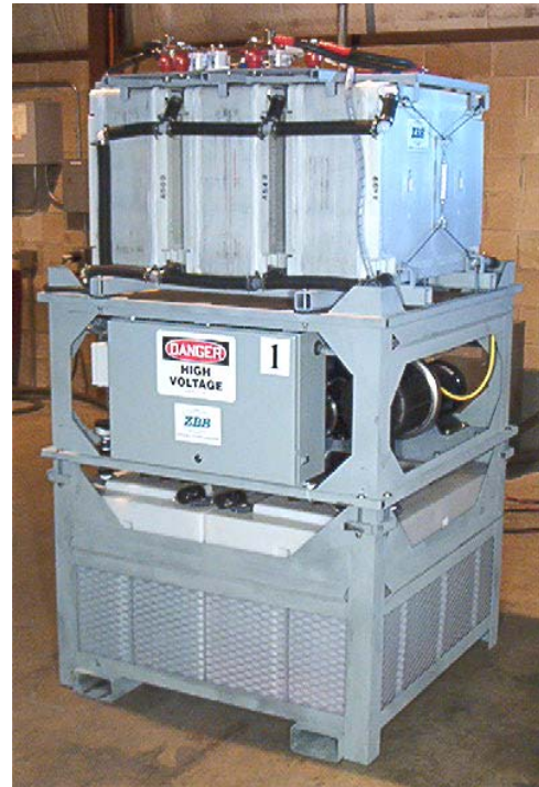
Figure 1. 50-kWh Z-BESS module.
